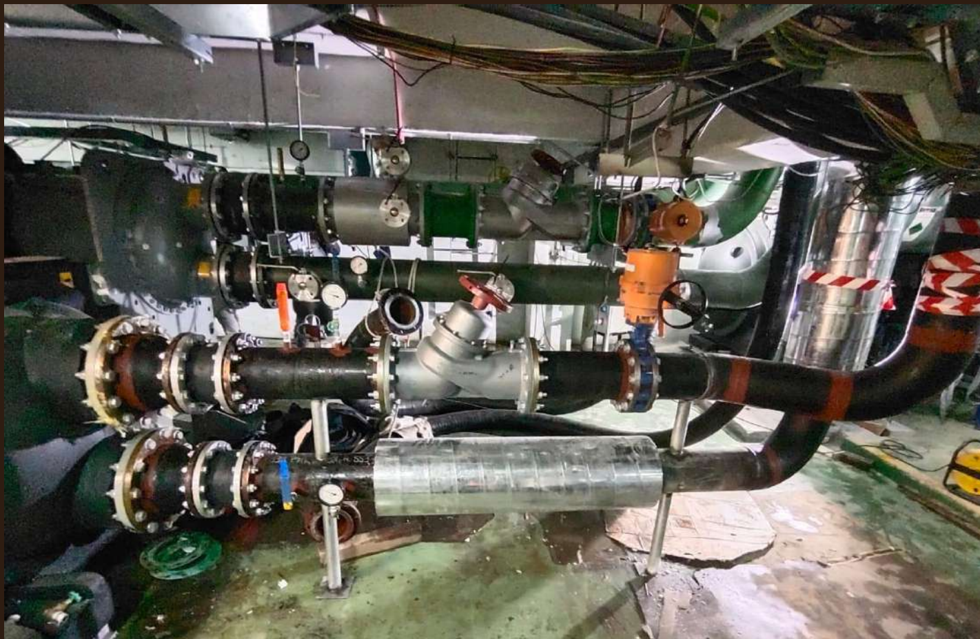
Chiller plant chilled water piping
