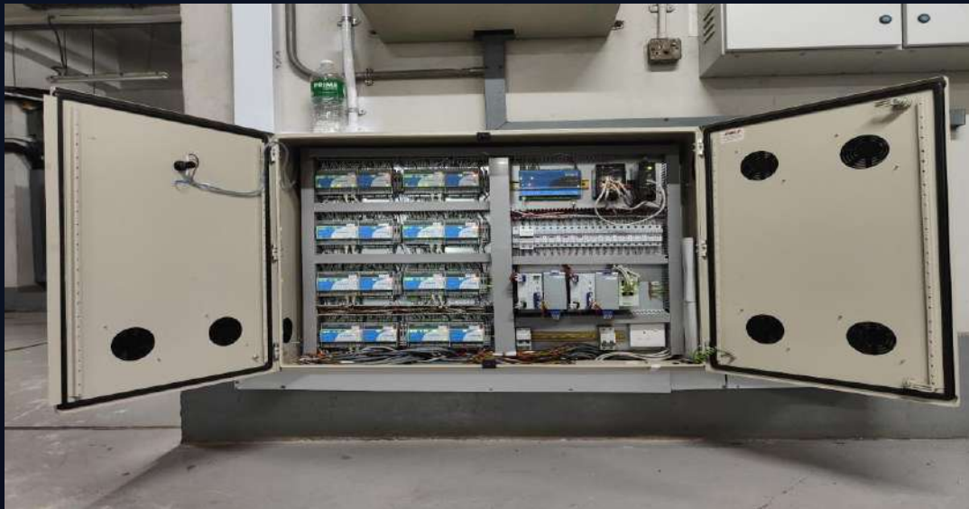
BMS control enclosure
