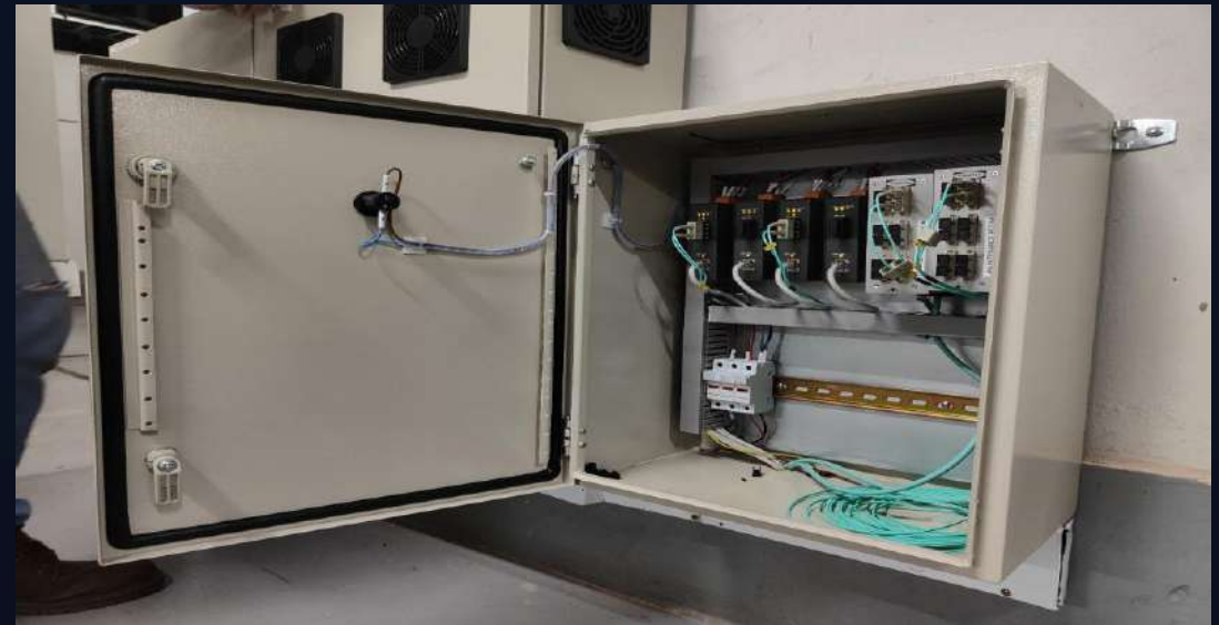
Field-wired BMS panel
