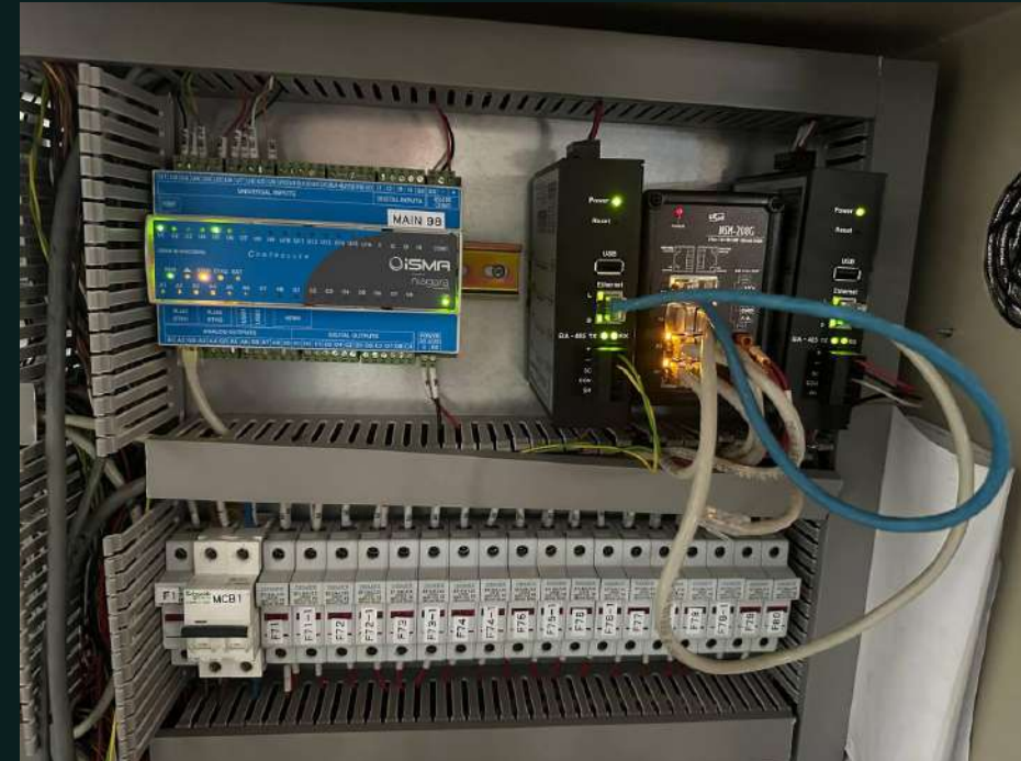
BMS controller cabinet interior · Power-Plus
